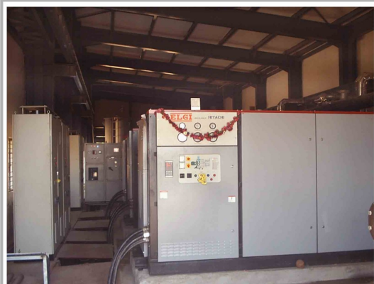
Elgi's oil free compressors at Karwar Naval base
