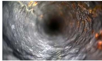
Real life problem 2 Corrosion of Piping
